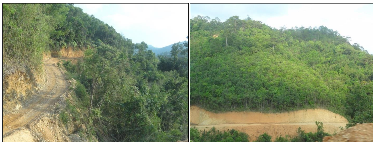
Figure 29. Road under construction (within Xe Sap NPA) with young fallow and bamboo forests without commercial timber by the sides.
